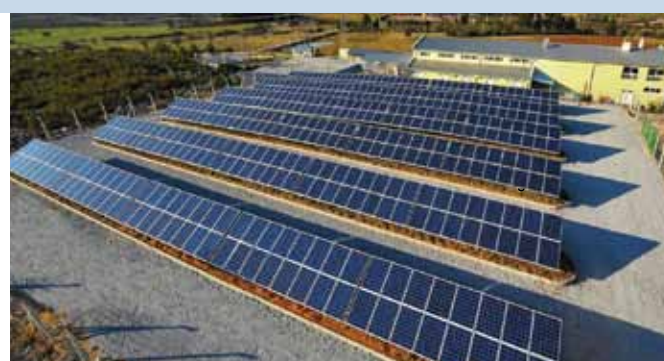
Fig. 4 - 105 kW grid-connected PV system in Muğla, Turkey.
