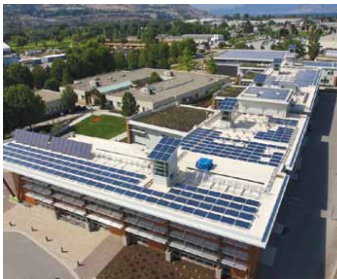
Fig. 1 - A 260 kilowatt solar PV rooftop system installed at the Okanogan College in British Columbia to meet the ambitious target for the living challenge and help train students in green construction practices (Photo: Skyfire Energy).
