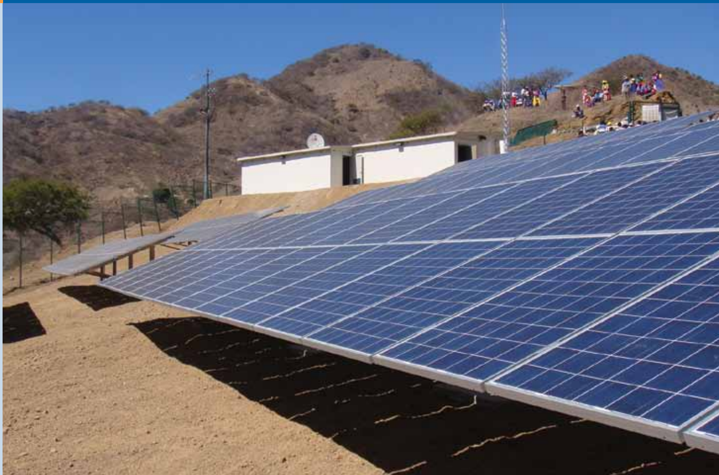
Fig. 2 - 50 kWp solar farm used for rural electrification in Nayarit, Mexico.
