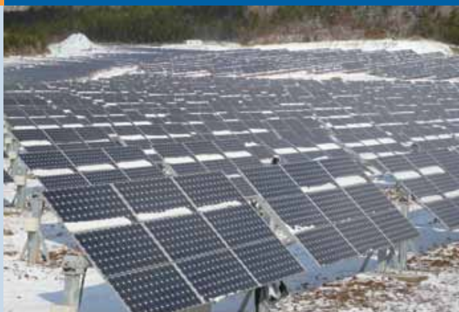
Fig. 3 – 3 MW PV power plant, Jeollanam-do, Korea.
