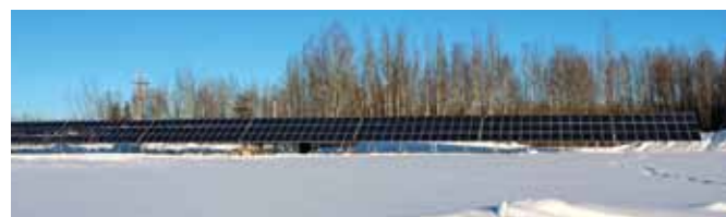
Fig. 2 - Fort Simpson is Northwest Territories Power Corporation largest diesel-powered community. This 61 kilowatt system (the largest North of 60 degrees in Canada) will help displace 15 000 litres of fuel annually and provide up to 8,5 % of the village's minimum power requirements during the summer (Photo: Skyfire Energy).
