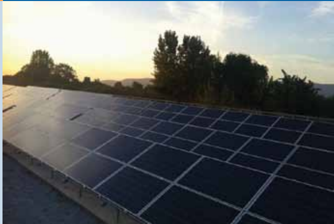
Fig. 5 - 96 kW grid-connected PV system in Bursa, Turkey.
