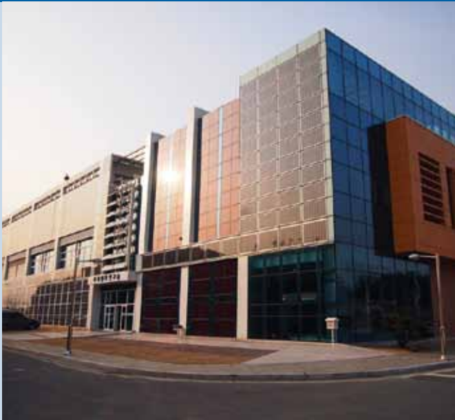
Fig. 1 – 111,2 kW BIPV system located at the Climate Change Research Building of the National Institute of Environmental Research, Incheon, Korea.
