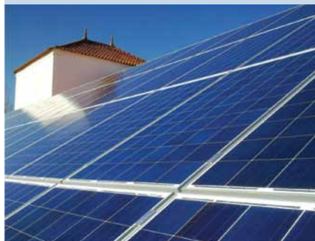
Fig. 3 - 60 kWp minigeneration project on the rooftop of a company in Portugal.
