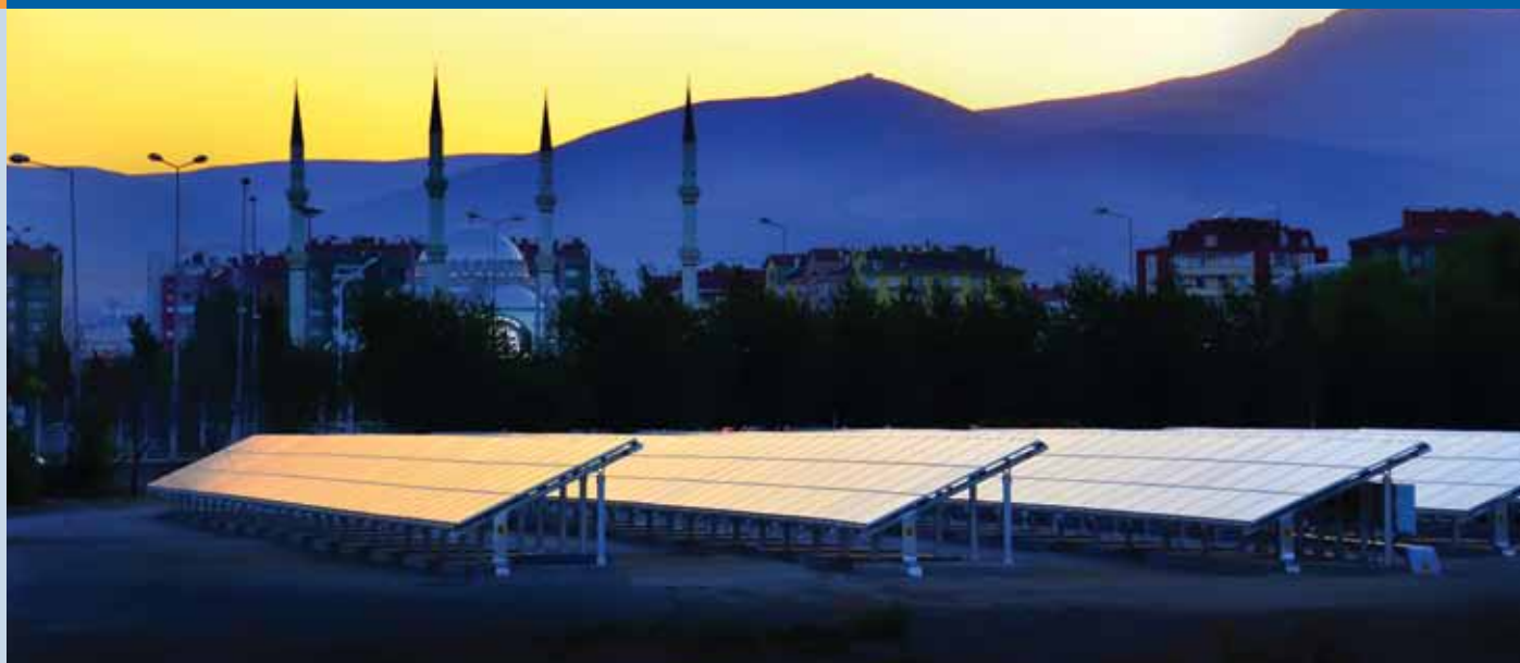
Fig. 3 - 200 kW grid-connected PV system in Konya, Turkey.
