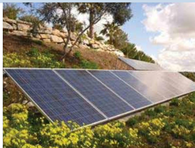
Fig. 2 - 4 kWp microgeneration project for a domestic house in Portugal.
