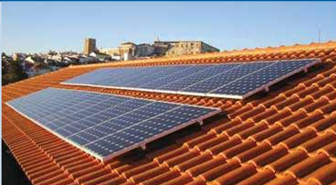
Fig. 1 - 4 kWp microgeneration project in a public health centre in Portugal.
