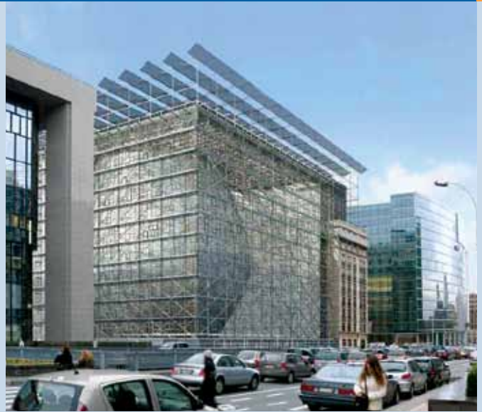
Fig. 4 – European Headquarters: Both the modern and the historical parts of the European Commission's new building, currently in construction, will be covered by an umbrella of photovoltaic panels.
