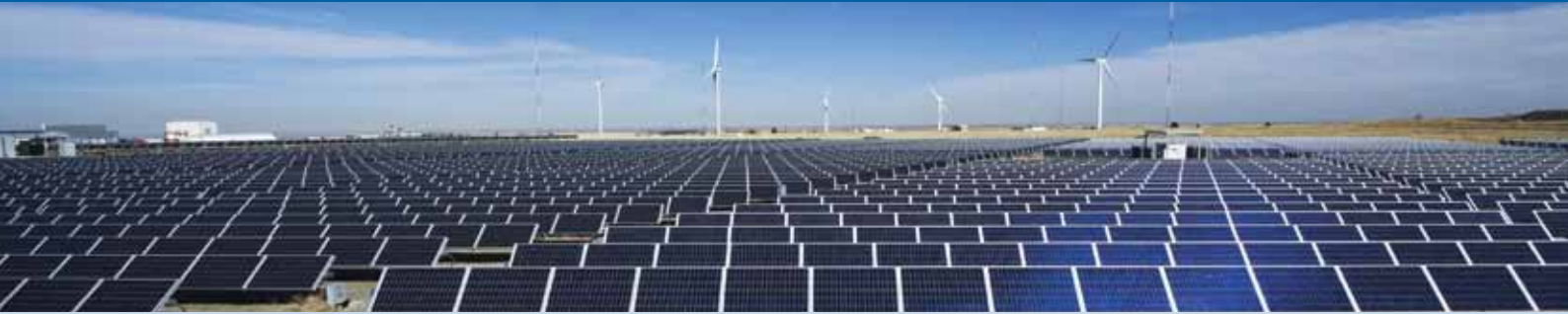
Fig. 1 - NREL's newest PV array at the National Wind Technology Center near Boulder, Colo., is an opportunity to study how ecosystems respond to renewable energy development and develop best management practices that re-establish habitat, minimize weed invasion, prevent erosion and protect wildlife. NREL's newest source of clean energy - a 1 megawatt solar array - is supplying laboratory researchers with more than carbon-free electricity. It's also an opportunity to examine a sensitive topic - the potential environmental impacts of large-scale renewable energy projects (Photo: Dennis Schroeder / NREL).
