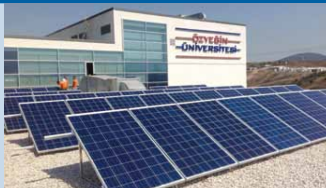
Fig. 1 - 13 kW grid-connected PV system in Özyeğin University, Istanbul, Turkey.
