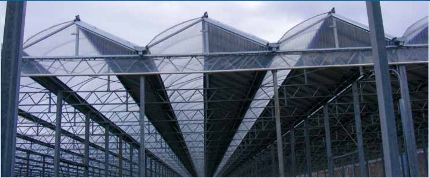
Fig. 1 – 3,0 MW Orsomarso PV Plant on a greenhouse at Cosenza (Photo: Hfv spa).
