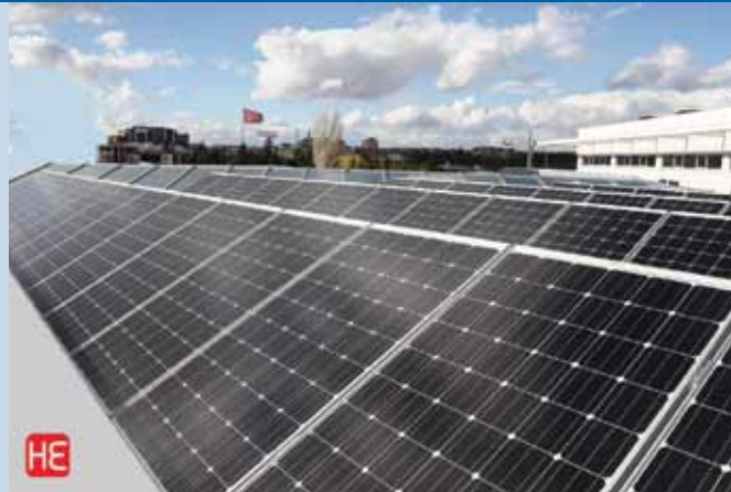
Fig. 6 - 95 kW grid-connected PV system in Eskişehir, Turkey.
