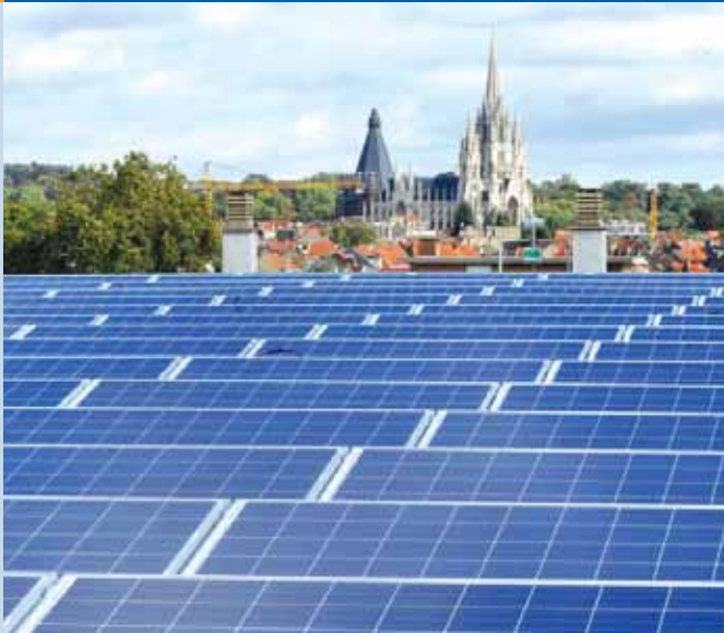
Fig. 2 – Brussels Port: The biggest urban PV installation in Belgium has been built in the port of Brussels: 1,2 MWp.
