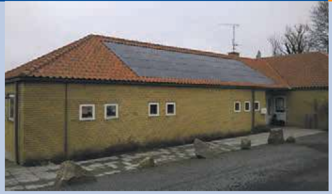
Fig. 4 - Roof integrated PV system by Storløkke holiday centre in Bornholm. A part of the PV Island Bornholm R&D project. Developed by Nielsen EI, Rønne.
