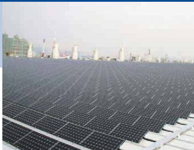
Fig. 2 - 3 MW roof mounted PV system at LG Electronics, Gumi-si, Gyeongsangbuk-do, Korea (Photo: Solar Today).
