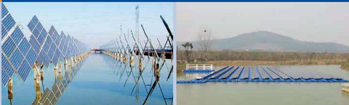
Fig. 2 - Fish-Pool PV and PV on Water Surface.
