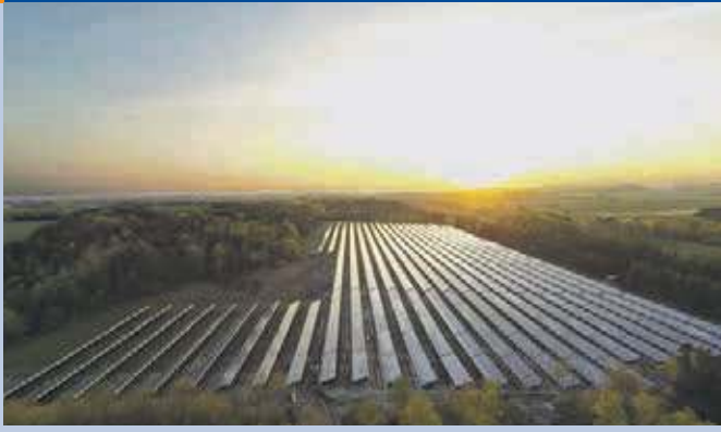
Fig. 3 - Sunset over a 2,38 MW PV park in Kollund. Developed by Sveigaard, Herning.
