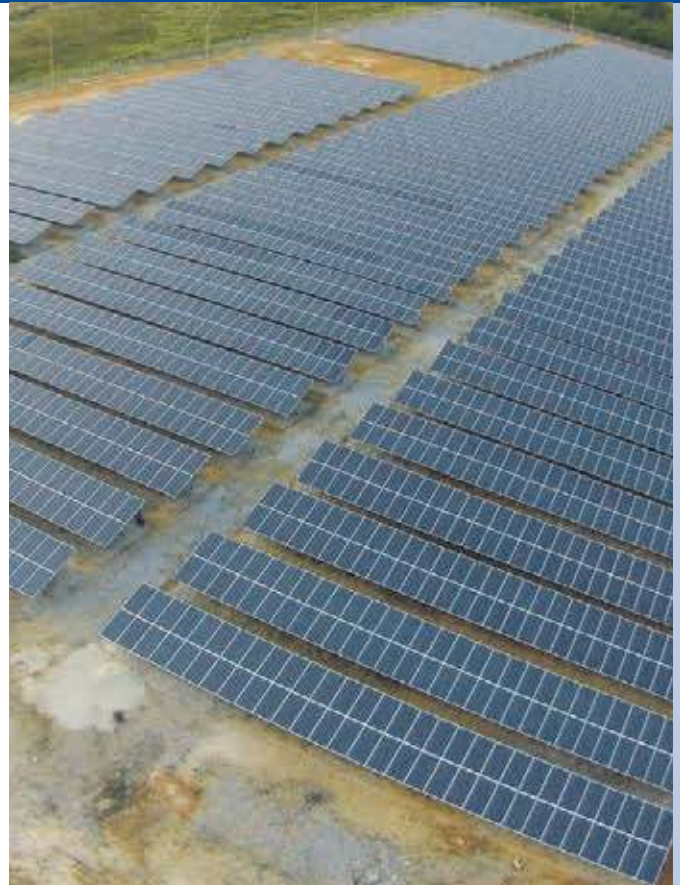
Fig. 1 - A PV farm of 1,764 MW in Kedah, Malaysia by Leaf Energy Sdn Bhd.
