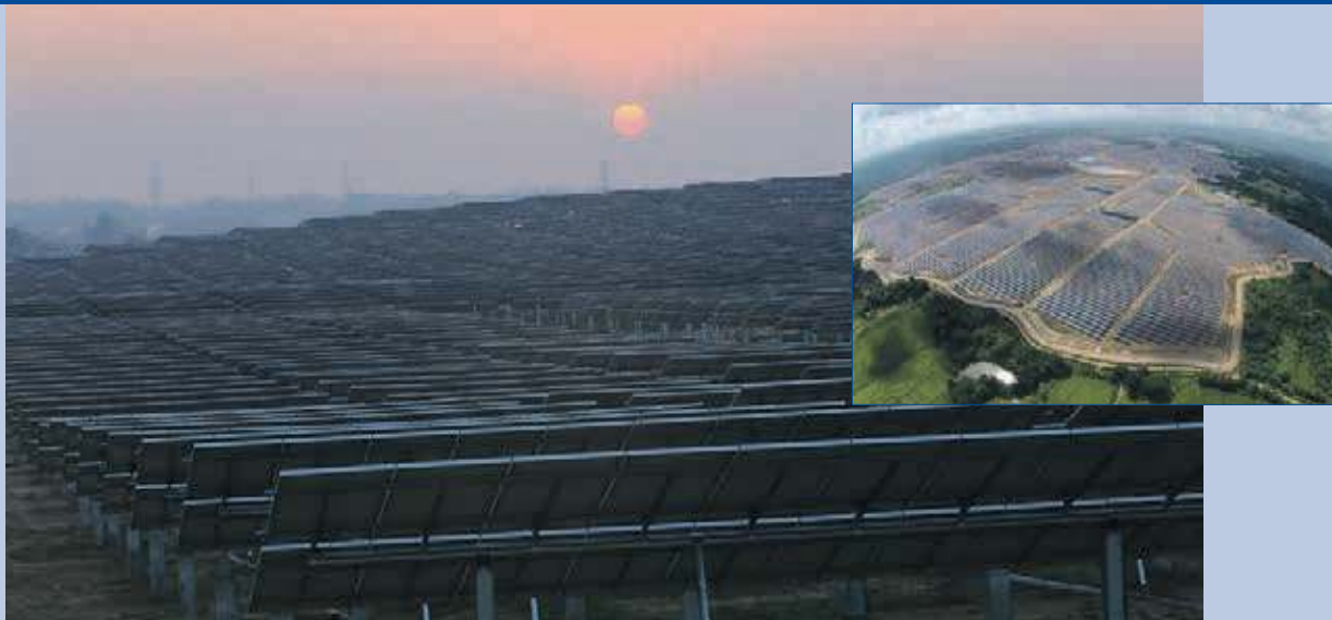
Fig. 3 - The Biggest SPP Project in 2015. This project has achieved COD since February 2015 in Lamphang province. Total installed capacity 126,396 MWp with Poly Crystalline Solar Cell, Solar Tracking System (Photos: Energy Absolute Public Company Limited).
