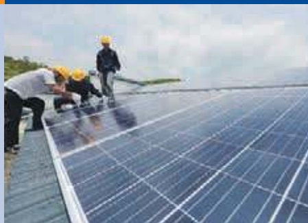
Fig. 4 - Technicians are installing PV system for a rural house in Guzhang county, Jiangxi province.
