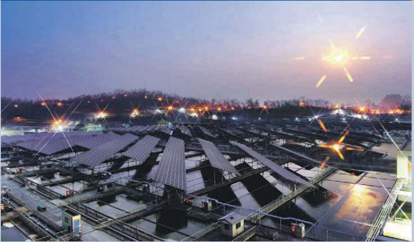
Fig. 3 - 5 MW PV power plant at Amsa Arisu Water Filtration Center, Seoul, Korea (Photo: Hankook-Ilbo).
