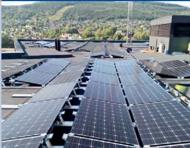
Fig. 2 - Omsorgsbygg Oslo installed a 130 kWp system at Økern Sykehjem (a home for elderly people). The power from the system is for self-consumption (Photo: Fusen AS).
