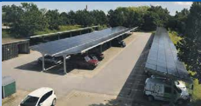
Fig. 1 - Car park with a 152 kWp PV system from the town hall in Fredensborg. Developed by Solar Park.
