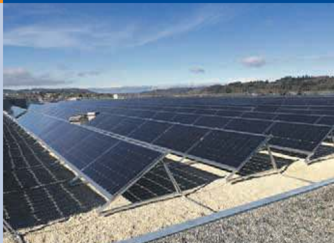
Fig. 2 - Self-consumption 658 kW PV system on a MIGROS supermarket with bifacial glass-glass modules, Schönbühl (Photo: Genossenschaft Migros Aare).
