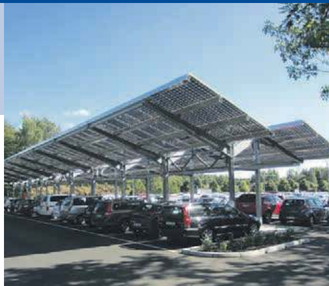
Fig. 3 - First stage on a planned 700 kW PV installation on roofs over a car parking, at Skaraborg Hospital (Photo: Johan Paradis).
