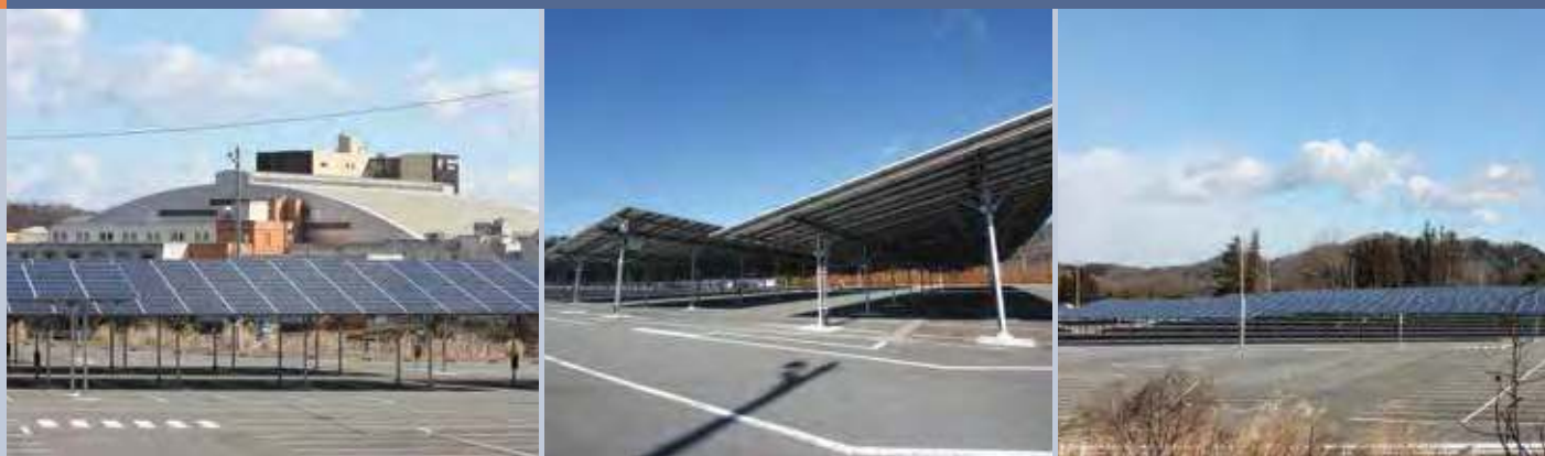
Fig. 3 - PV System for a Parking Lot (Spa Resort Hawaiians) (Iwaki City, Fukushima Prefecture). 2.1 MW Multicrystalline silicon PV module (by Yingli, 275 W x 7,627 modules).
