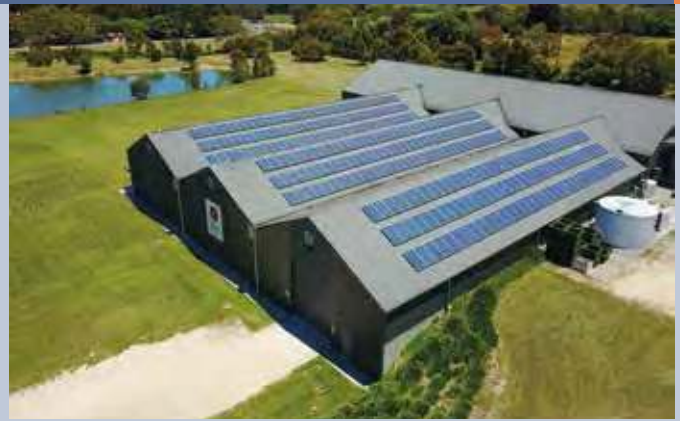
Fig. 4 - Wicks Winery Estate. Woodside, South Australia. 80 kW system sold and installed by Venergy Australia (Photo: Matt Wilkins).
