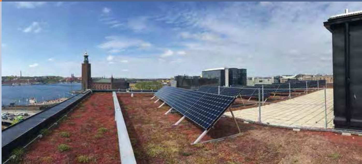
Fig. 3 - PV system on green roof, SPP, Stockholm - 32 kW (Photo: Solkompaniet).
