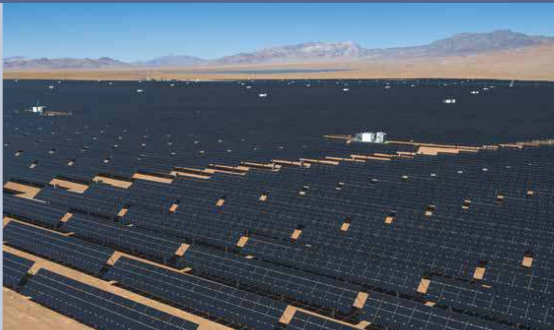
Fig. 3 - Large PV Plant. 141 MW Luz del Norte PV Plant (First Solar) located at Copiapó, Atacama Region, Chile.
