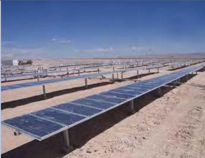
Fig. 1 - Calama Solar 3. This 1 MW power plant provides electricity to the industrial facilities of División Chuquicamata (the largest open-pit copper mine in the world).
