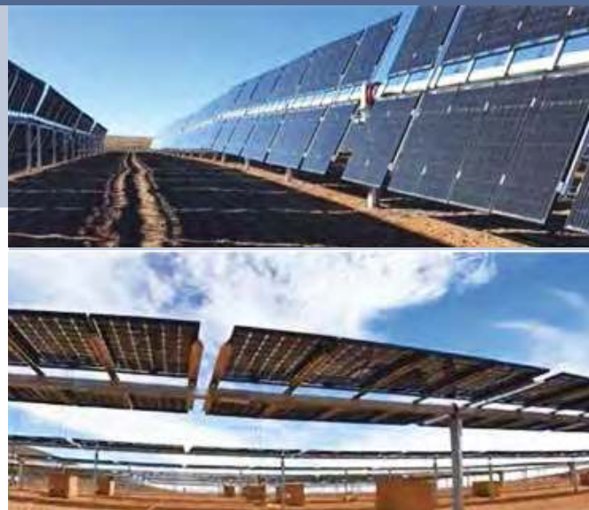
Fig. 2 - Bifacial modules Installed by EGP on one-axis sun trackers manufactured in Italy (Photo: ENEL Green Power).
