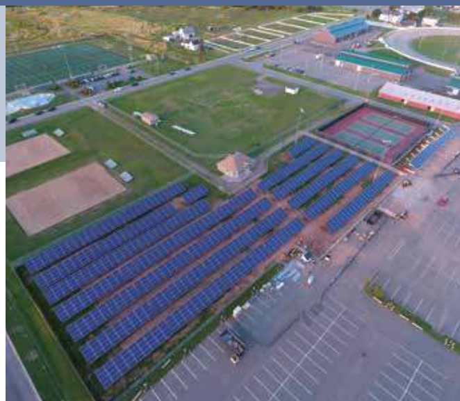
Fig. 2 - Credit Union Place Smart Solar Storage System – 494 kW p , Summerside, PEI.
