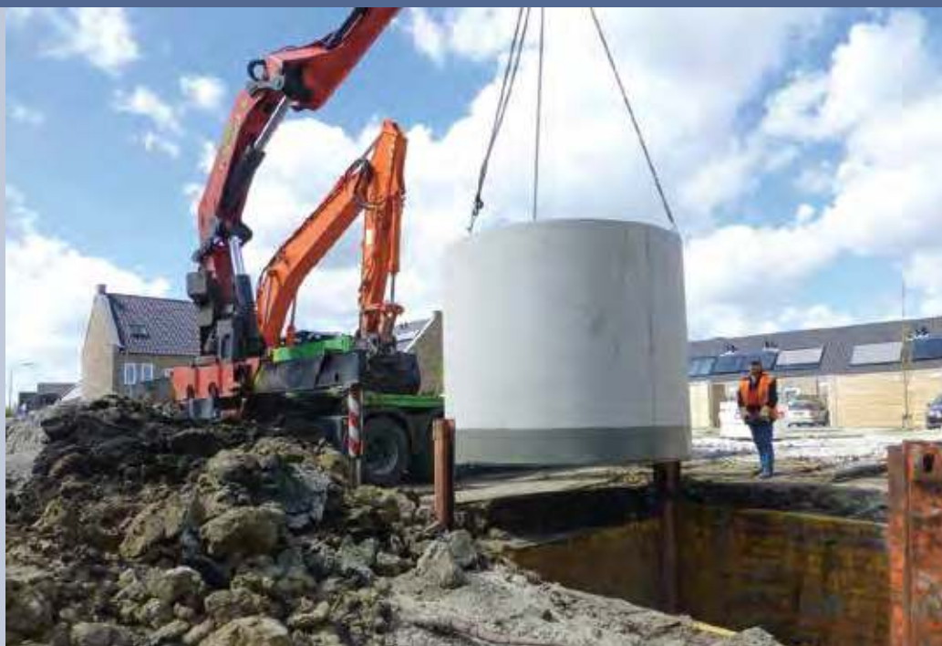
Fig. 2 - Installation of ice/water storage tank Goes, Province Zeeland, courtesy of Marsaki (Photo: Marsaki & RWS partner in wonen).
