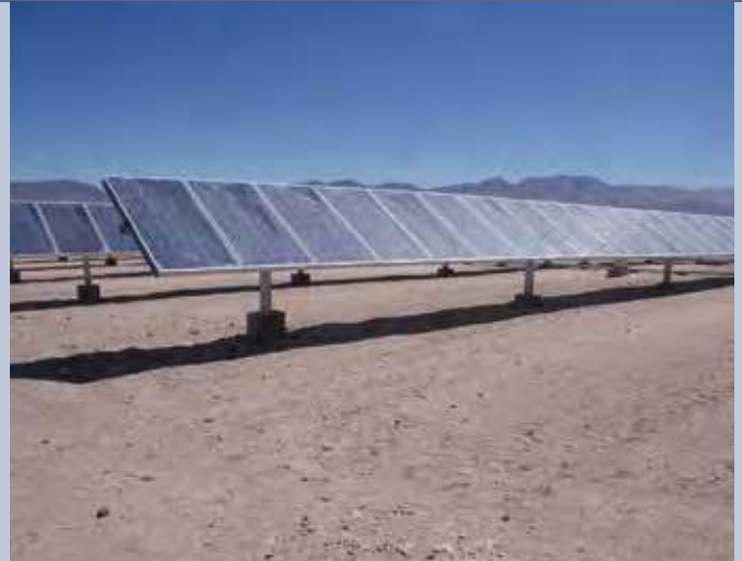
Fig. 2 - Calama Solar 3. The excellent local radiation conditions, in combination with the one-axis tracking systems, makes this 1 MW plant to deliver an outstanding annual generation of 2900 MWh (data April 2012 - March 2013).
