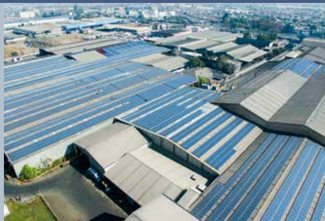
Fig. 5 - CINTAC PV rooftop plant located in Maipo industrial sector, south of Santiago city, grid connected 2,78 MWp.
