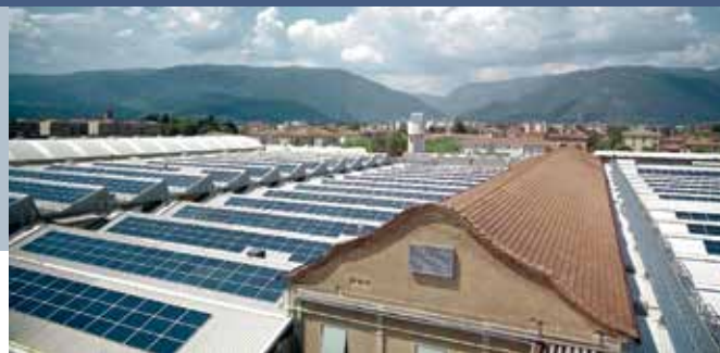
Fig. 4 - 1 MW PV plant on the BAXI roofs in Bassano del Grappa, which uses monocrystalline FU270P modules (Photo: FuturaSun).
