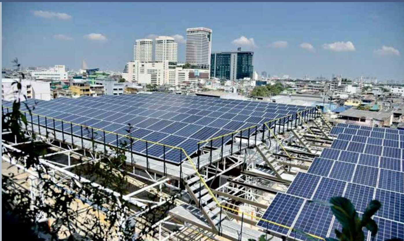
Fig. 1 – The 75 kW PV rooftop project installed over the parking building of the Department of Alternative Energy Development and Efficiency, Ministry of Energy of Thailand. The project aims to introduce demand-side management program to increase renewable energy consumption in the building using Building Energy Management System (BEMS) to balance between generated power and electricity demand, and to cut peak demand of building electricity need (Photo: DEDE).
