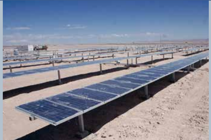
Fig. 2 - Calama Solar 3. This 1 MW power plant provides electricity to the industrial facilities of División Chuquicamata (the largest open-pit copper mine in the world) in Chile.
