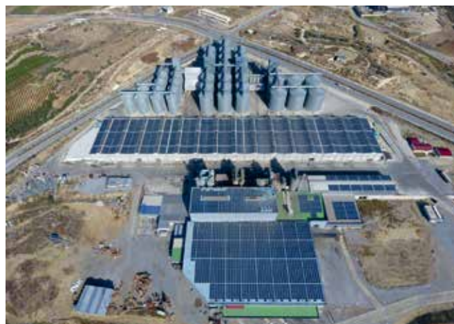
Fig. 2 - Commercial rooftop PV power system at Tiryaki Agro Company in Mersin (4.24 MW) [23].
