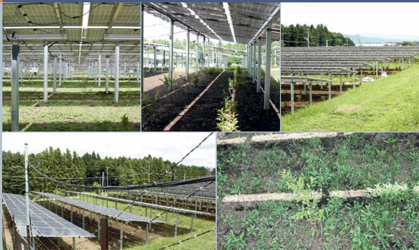
Fig. 2 - Large-scale PV systems on farmland (Gotemba PV Power Plant No. 1 & No. 2) (Gotemba City, Shizuoka Prefecture). "SPLITMAX" PV modules using half-cut cells (by Trina Solar) (335 W).
