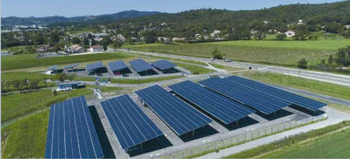
Fig. 1 – Urbasolar's 854 kWp solar canopy over the employee parking lot at the NTN-SNR Cévennes St. Privaden site in France (Photo: Urbasolar/M. Colin).
