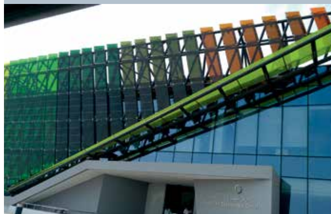
Fig. 6 - Construction work from ONYX SOLAR for the installation of BIPV in DEWA's building for R&D (Dubai).
