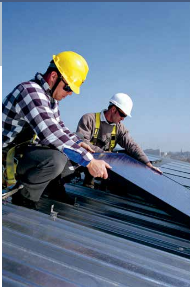
Fig. 2 - Workers install PV panels on Natatorium in Atlanta, Georgia; Georgia Institute of Technology.
