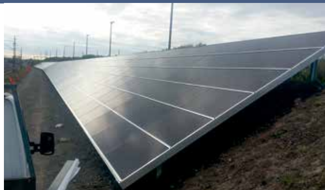
Fig. 1 - PV system for Øresundsbroen (the bridge between Denmark and Sweden). The power of the system is 255 kWp. System delivered by Helge Andersen, Solarpark DK A/S, Denmark.
