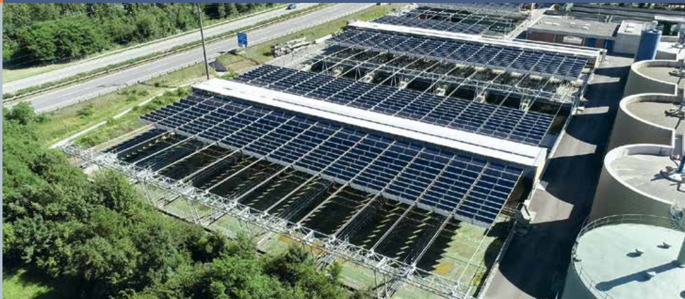
Fig. 5 - dhp has realized the world's first solar folding roof across a sewage infrastructure, a consistent double use of already sealed land for solar power generation in urban infrastructures and with 100% self-consumption. Following a pilot plant with the HORIZON solar folding roof, the system was extended to a capacity of 643 kW in 2018 (Photo: © dhp technology).
