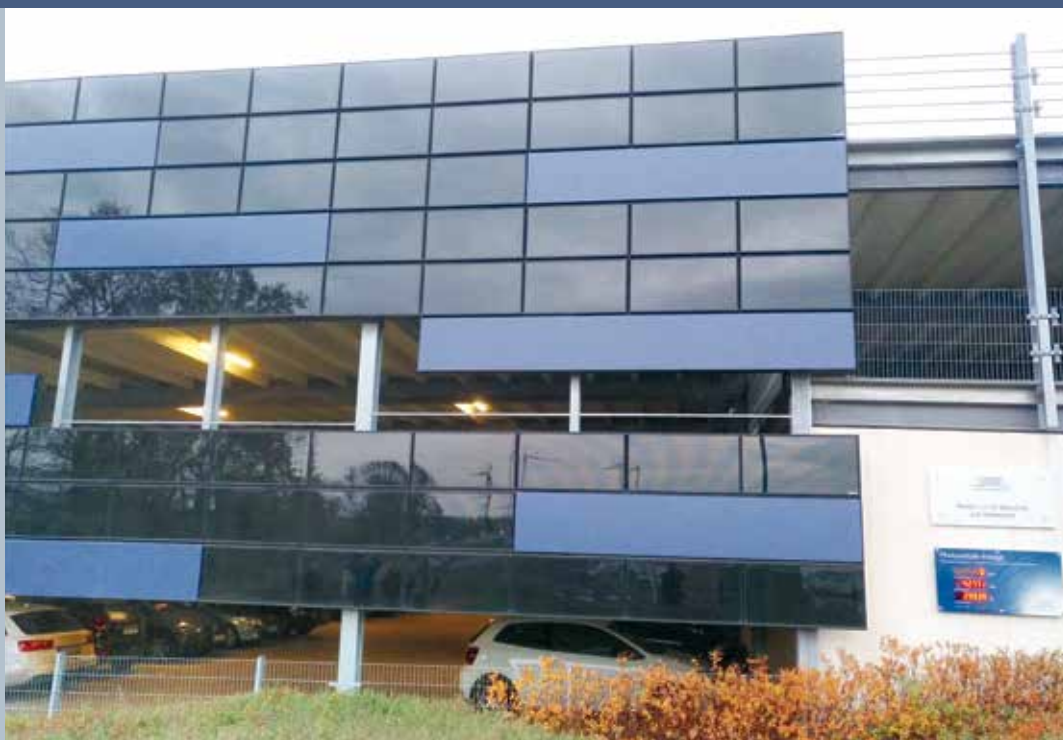
Fig. 5 - Building integrated PV facade on a multi-storey car park (Photo: © PJ / Klaus Prume).
