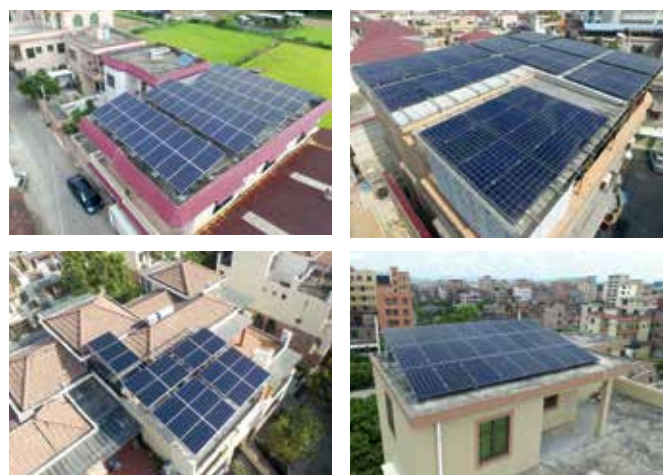
Fig. 3 - PV Home Systems (Photo: Solarq).
