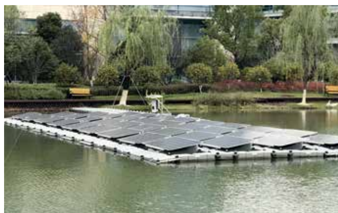
Fig. 2 - Demonstration floating PV system in China (Photo: taken at GCL Future Energy Exhibition Hall, Suzhou, China, J. Stein, SANDIA).
