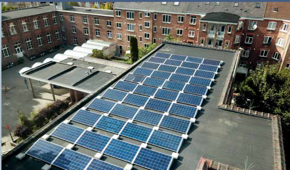
Fig. 2 - PV Project at School: Ecole St. Anne in Brussels, realized through crowdfunding from school and parents. Installation in 2018.
