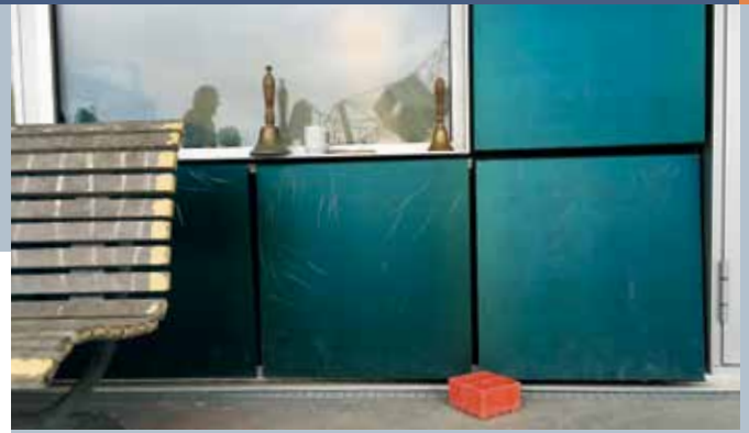
Fig 6 – BIPV installation at the Copenhagen International School, Copenhagen, Denmark. BIPV developed by Anders Smith and realized in 2017.
