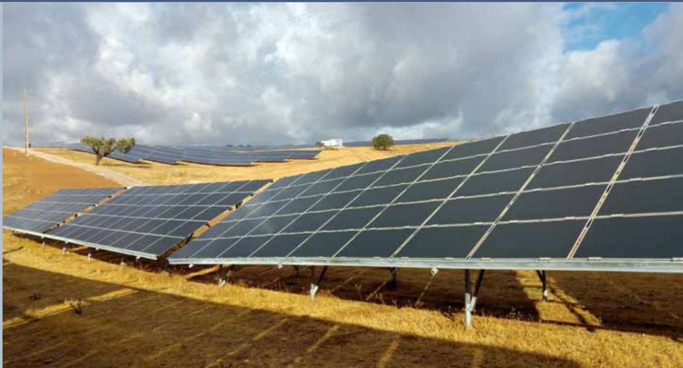
Fig. 1 – 4,1 MW CSF MONTES NOVOS PV plant at Estremoz (Photo: Edgar Santos).
