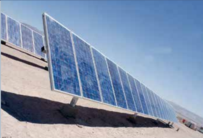
Fig. 1 - Calama Solar 3. The excellent local radiation conditions, in combination with the one-axis tracking systems, makes this 1 MW plant to deliver an outstanding annual generation of 2 900 MWh.
