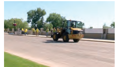
Public Works employees install the removable panels to Austin’s flood wall to prepare for high waters.
