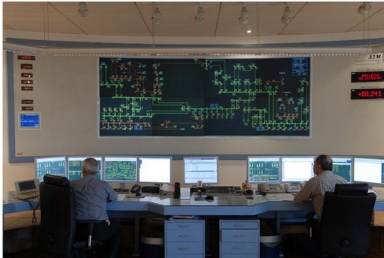
Figure 2.3: Control center of Cyprus as typical but relatively small control center
