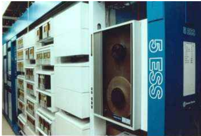
Fig. 5-16. The 5ESS® switching system was manufactured initially by Western Electric, with its initial installation in 1982, and later by Lucent Technologies. It is an all-digital switching system with time-slot interexchange. [Photo courtesy of Alcatel-Lucent USA Inc. / Bell Labs.]
