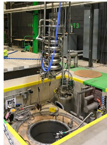
Figure 5.7: Upgrade cavity is being loaded into the cryostat.
