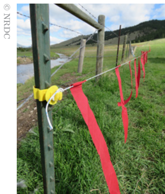
Poly wire should be tied off to an insulator on a T-post at the starting point for installation.
