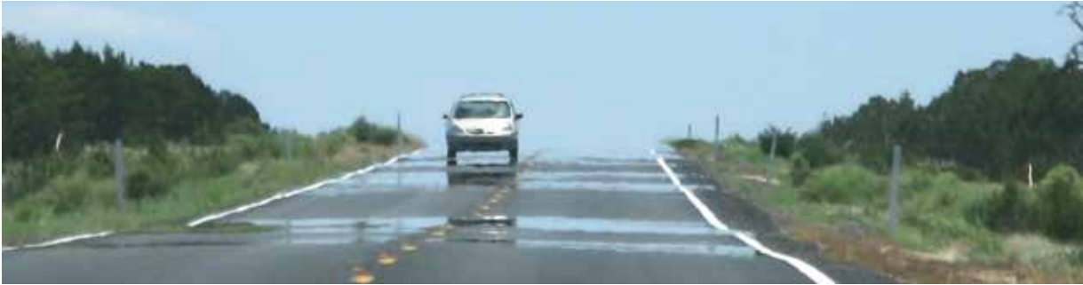
Extreme temperatures can cause roadways to buckle and crack. Photo credit: Adobe Stock
