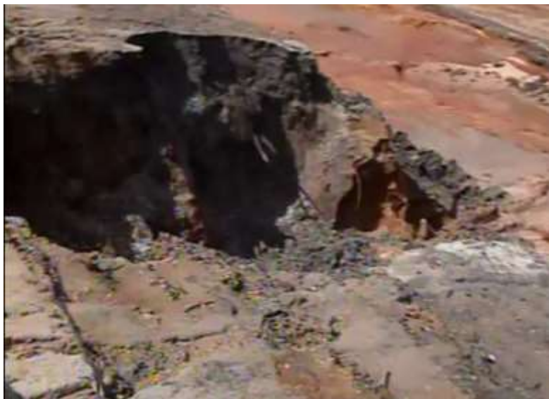
Figure 12. Photos of Sinkhole on Upstream Slope of Dam Following Breach Development. See Figure 7 for Approximate Location on Cross Section.
