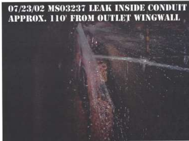
Figure 10. Photo of Leak Discharging into Conduit Approximately 110 Feet from the Outlet Wingwall. See Figure 7 for Approximate Location on Cross Section.
