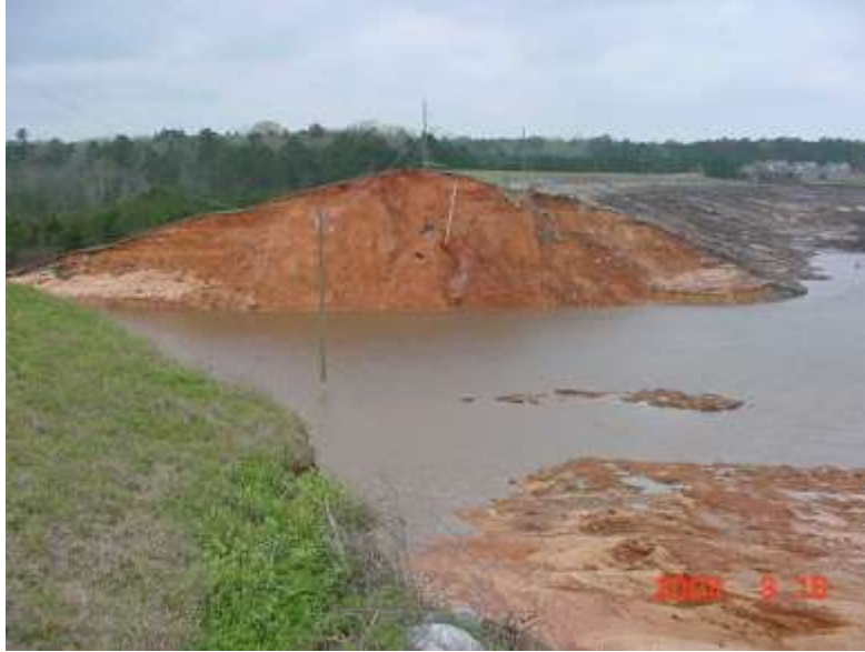
Figure 3. Photo of Dam Breach from Upstream Slope.
