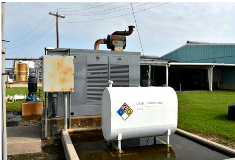
Inundated power generator at the Arkema facility following the chemical disaster. Source: U.S. Chemical Safety and Hazard Investigation Board
