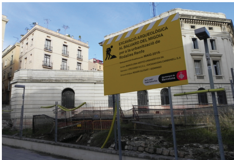
Figure 14. Works on the Bastion of Noon placed on the frontier between the neighbors of Barceloneta and La Ribera during 2014-2015. Ana Pastor.
