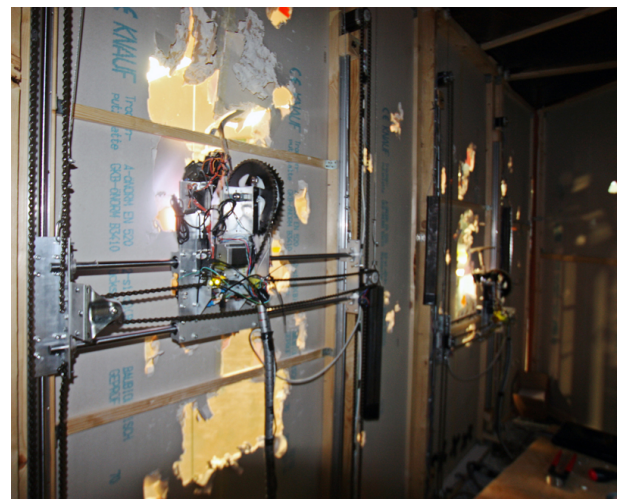
Figure 2: Robot gantries are attached to walls.
