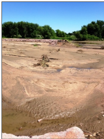
Figure 21 – June 2015: Trail Damage at Hanson Trailhead
