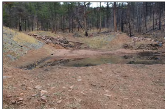
Evidence of Erosion
