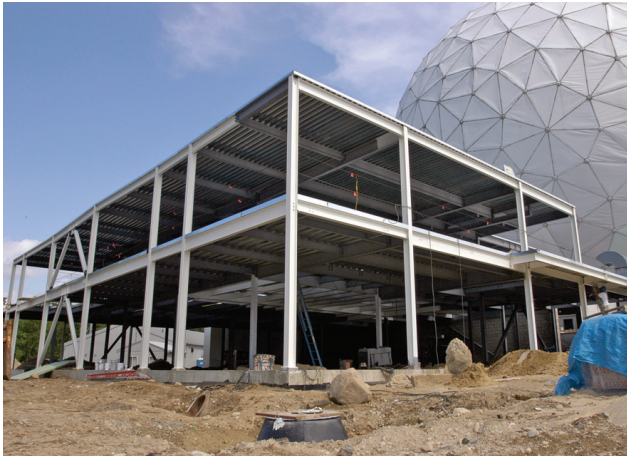
FIGURE 1. Construction of the 10,000-square-foot HUSIR transmitter equipment shelter took place in 2005. High-voltage modulators and VEDs occupy the ground floor; waveguide, combiners, and multiplexers occupy the mezzanine level. The floor area and positioning of the vertical columns were dictated by the need to keep up to 17 superconducting magnets at least two meters away from each other and from the nearest column.
