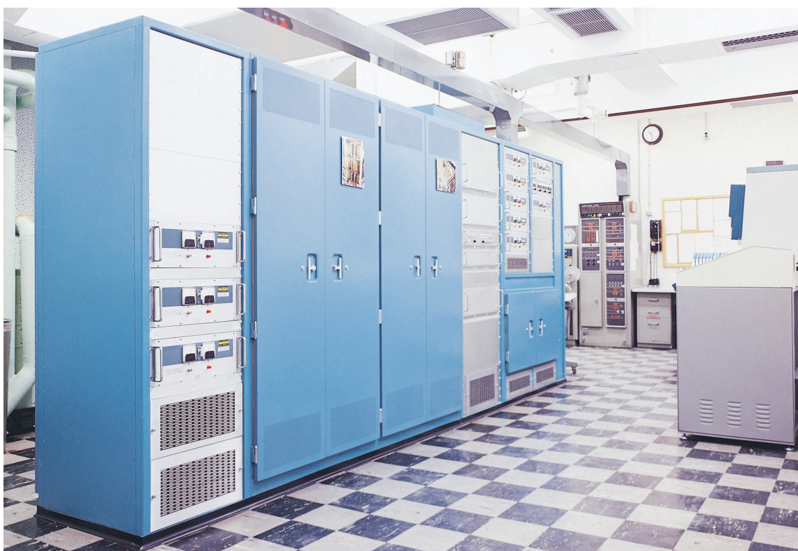
FIGURE 8. The FDP facility at Lincoln Laboratory in 1970, which included a Univac 1219 general-purpose host computer. The arithmetic/logic unit incorporated a full 18-bit, twos-complement adder/subtractor, supported all Boolean functions, and included linkages for extended-precision calculations. The 18 \times 18 -bit four-quadrant multiplier was based on a modified Booth's algorithm, and was implemented as a full combinatorial array using single-bit adders.
