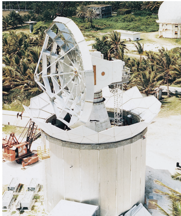
FIGURE 17. Construction of the MMW (millimeter-wave) radar and radome on Roi-Namur, Marshall Islands. The heavy structure of the dish is needed to achieve the surface tolerance required for the short wavelengths of the radar.
