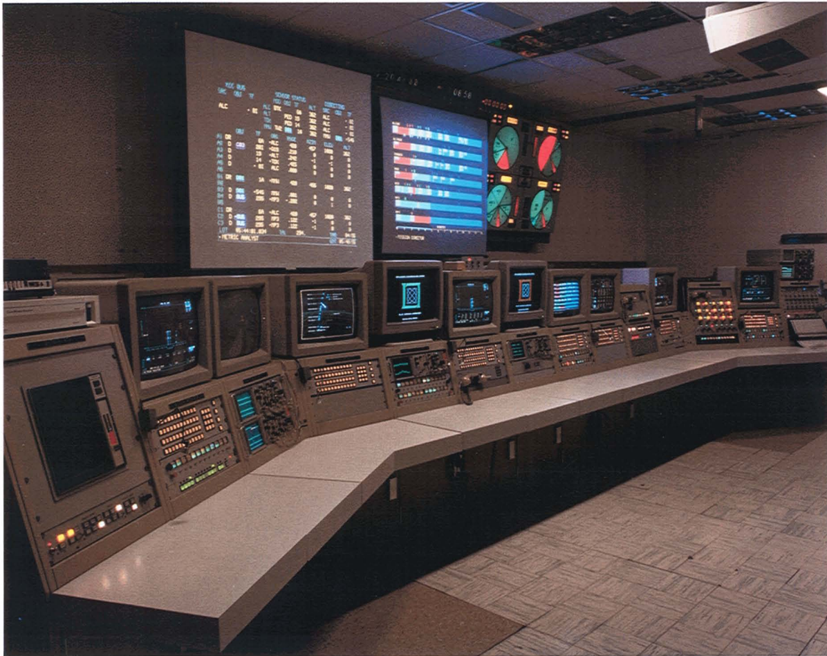
Fig. 6—The KREMS Control Center's operator console.
