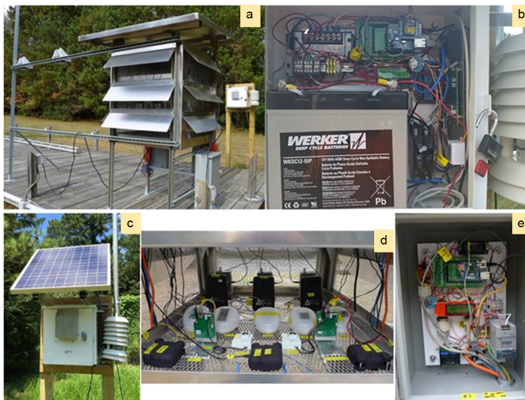
Figure 1. CAIRSENSE field equipment, including (a) SAFT instrument enclosure, (b and c) solar-powered WSN node, (d) interior of SAFT instrument shelter, and (e) WSN node utilizing 120 V (nominal) AC electricity.
