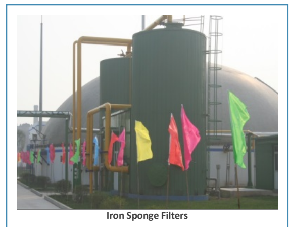
Biological H 2 S Scrubber
