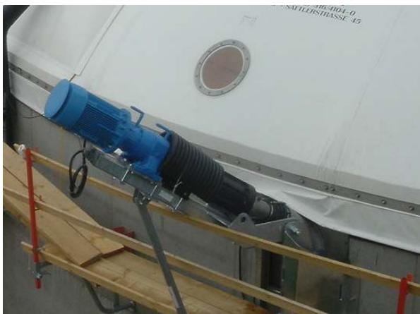
Side Mounted Digester Mixer and Tank View Port
