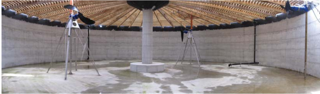
Complete Mix Digester Tank Showing Freestanding Mixers, Wooden Desulfurizers and Center Pier Column
