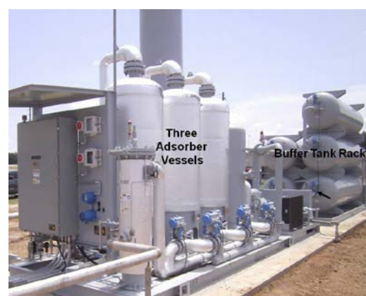
Biogas Upgrading System at GA Lagoon Based Digester
