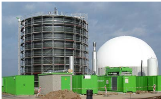
CSTR Complete Mix Digester, Inflatable Gas Storage and Containerized CHP Units
