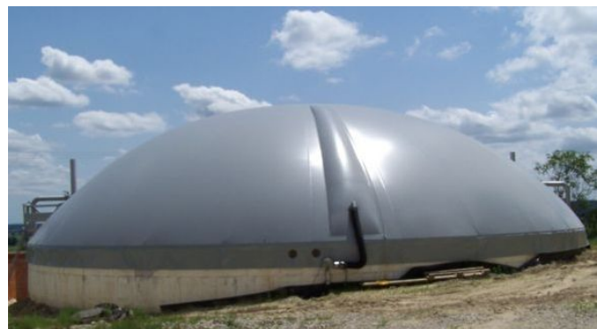
Gas Storage Dome Showing Inflation Hose
