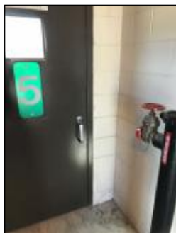
Finding 298053 Additional Photo
