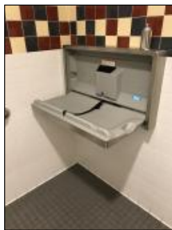
Finding 299281 Additional Photo
