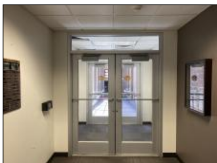
Finding 299595 Additional Photo
