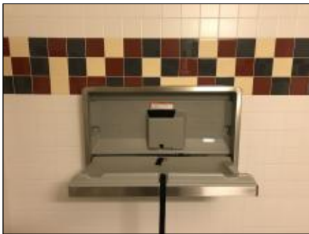
Finding 299274 Additional Photo
