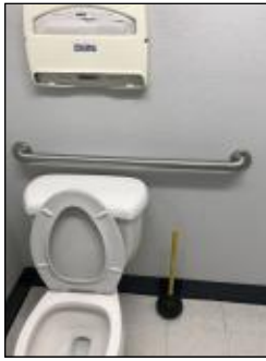
Finding 291397 Additional Photo
