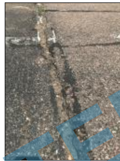
Finding 299370 Additional Photo
