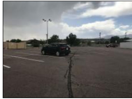
Finding 299327 Additional Photo
