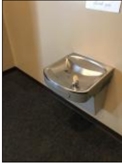
Finding 299369 Additional Photo
