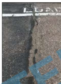
Finding 299332 Additional Photo
