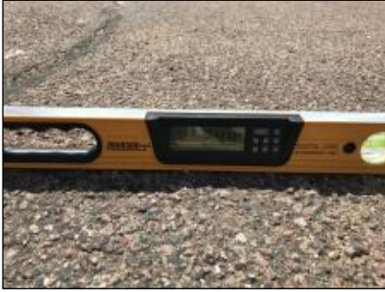
Finding 299371 Additional Photo
