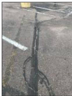
Finding 299332 Additional Photo
