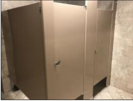
Finding 299362 Additional Photo
