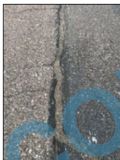
Finding 299332 Additional Photo
