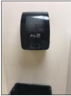
Finding 299335 Additional Photo
