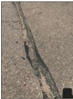
Finding 299370 Additional Photo
