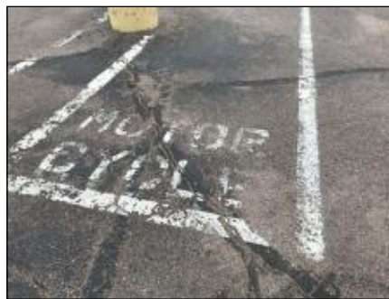
Finding 299332 Additional Photo
