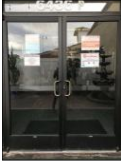
Finding 299334 Additional Photo
