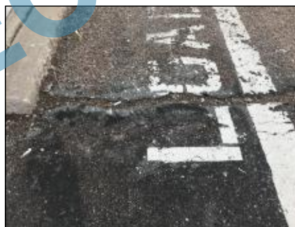
Finding 299332 Additional Photo
