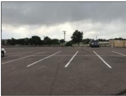
Finding 299327 Additional Photo
