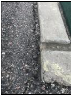
Finding 299331 Additional Photo
