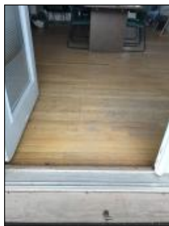
Finding 299285 Additional Photo
