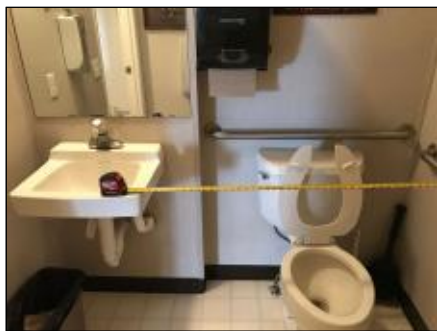
Finding 299290 Additional Photo
