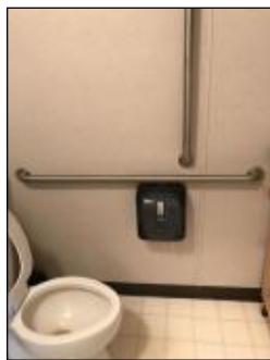
Finding 299291 Additional Photo
