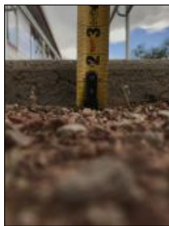
Finding 299300 Additional Photo
