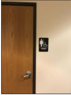
Finding 299248 Additional Photo
