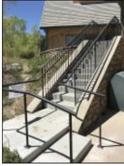
Finding 299269 Additional Photo
