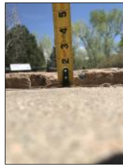
Finding 299246 Additional Photo
