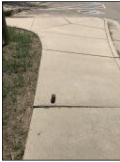
Finding 299246 Additional Photo
