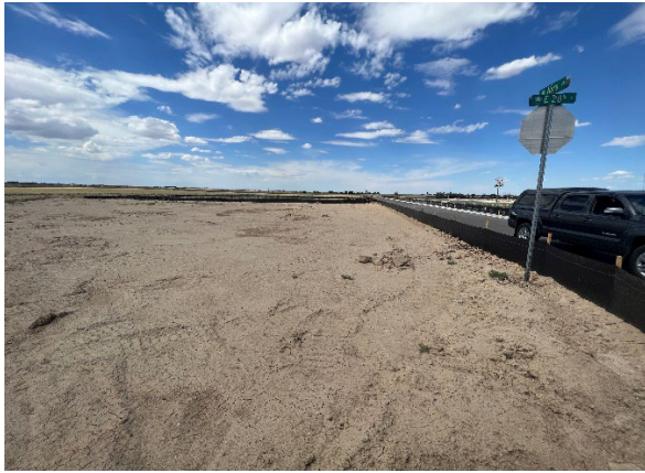
Photo 7: Grading activities and newly paved roads and sidewalks present on the eastern portion of Subject Property.
