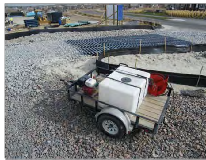
Photograph VTC-2. A vehicle tracking control pad with wheel wash facility. Photo courtesy of Tom Gore.
