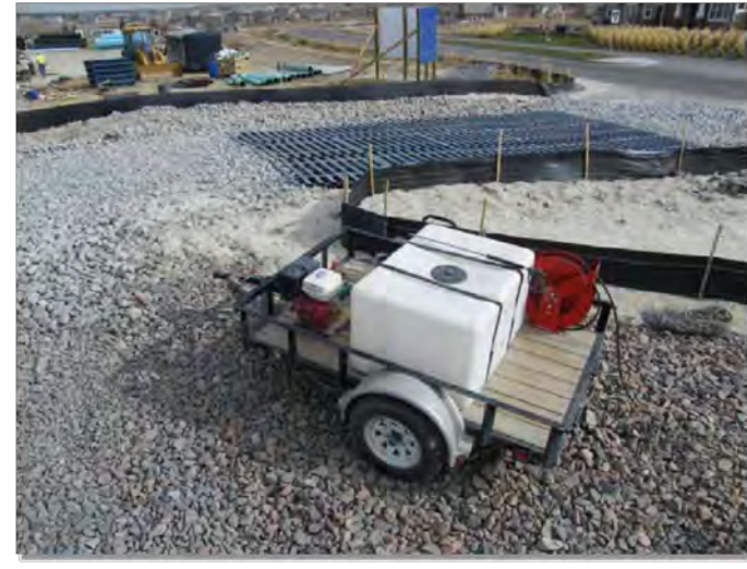
Photograph VTC-2. A vehicle tracking control pad with wheel wash facility. Photo courtesy of Tom Gore.
