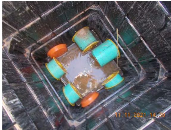
Distribution box for STA
