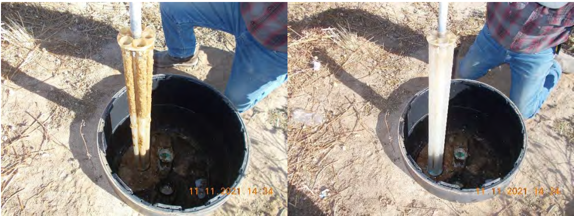
Effluent Filter – Before & After Cleaning
