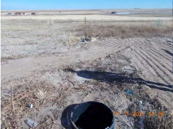
Looking east from tank to distribution box
