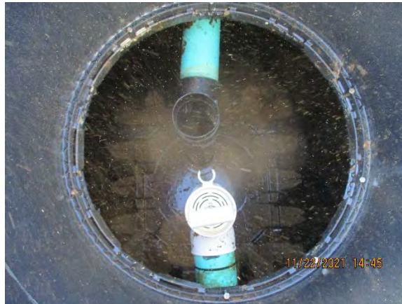
Access Port after pumping
