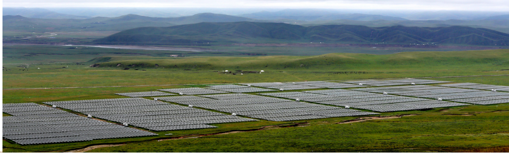
▼ 甘南太阳能光伏发电。刘铁军 摄 A glimpse of Gannan's solar power facilities
