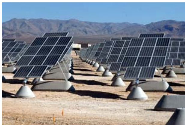
Figure 1. Gen 2 solar modules on single axis trackers at Nellis Airforce Base, Nevada USA.
