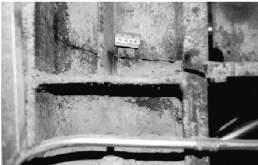
Figure 6.8. Example of a welded steel connection that fractured in the 1994 Northridge Earthquake. Notice that the weld between the flanges experienced a tensile crack that extended across the web of the steel column. Prior to this earthquake, it was generally believe that mild structural steel would ductily bend, but that it would never fracture. .
