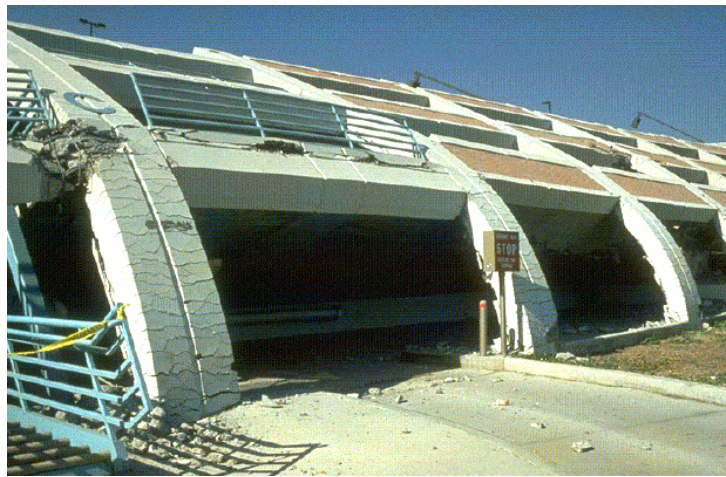
Figure 6.17. Example of ductile deformation of concrete columns from the 1994 Northridge earthquake. Adequate spiral reinforcing resulted in more ductile behavior than was shown in Figure 6.14. Unfortunately, the structure had other inadequacies that led to collapse as is shown in Figure 6.17.
