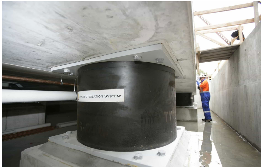
Figure 6-22. Base Isolated structure. The large black cylinder is one of many rubber/steel plate composite isolators that supports the weight of the building. The isolators are stiff in compression and flexible in shear. The concrete wall behind the engineer is the safety stop. The ground floor of the building is a massive reinforced concrete element that ensure that the ground floor moves as a rigid block.
