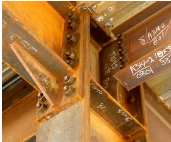
Figure 6.9. Post Northridge Special Moment Resisting connection (welded and bolted) in one direction and simple connection in the orthogonal direction
