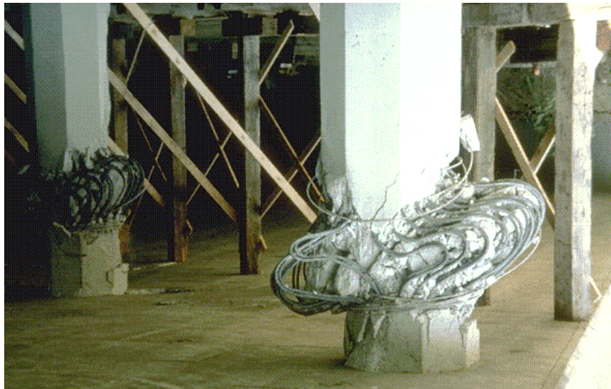
Figure 6.15. Example of a nonductile concrete column failure on a freeway bridge during the 1994 Northridge earthquake. The column was fractured by horizontal shear, the concrete fell away, and then the weight of the bridge deck caused the rebar to buckle. This failure could have been avoided by adding more spiral reinforcing loops radially around the column to make it more ductile as is seen in Fig. 6.16.
