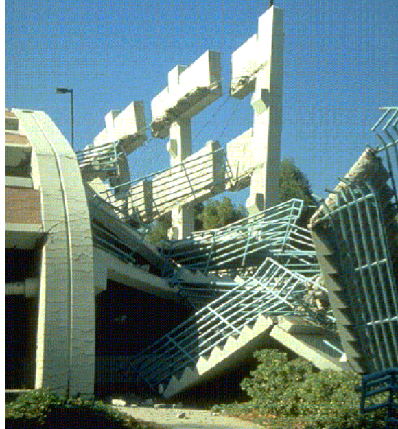
Figure 6.18. Despite the ductile behavior of the concrete columns, this parking structure collapsed because the floor slabs were not adequately connected to the rest of the structure. That is, the beams and columns were ductile, but the connections between these elements were not.
