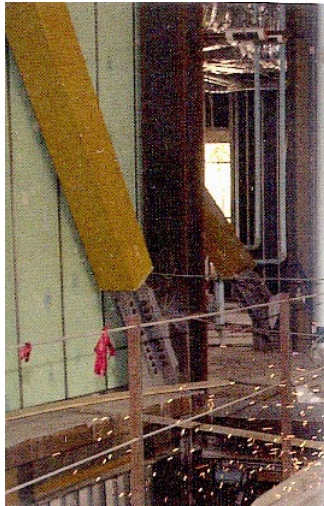
Unbonded Brace in the Broad Center
