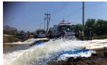
Drain pump car
