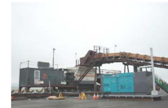
Intermediate treatment facility of mixture (sorting and crushing)
