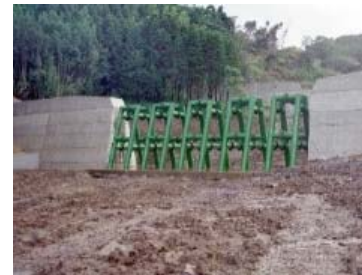
Driftwood Catching Check Dam
