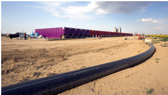
Surface frack water pipeline in Weld County
