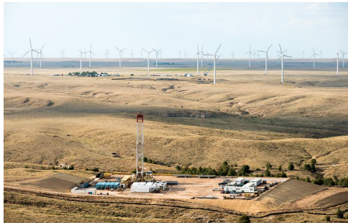
Constructed well pad with drilling rig in the Niobrara Shale. Source: Carrizo Oil & Gas Inc.
