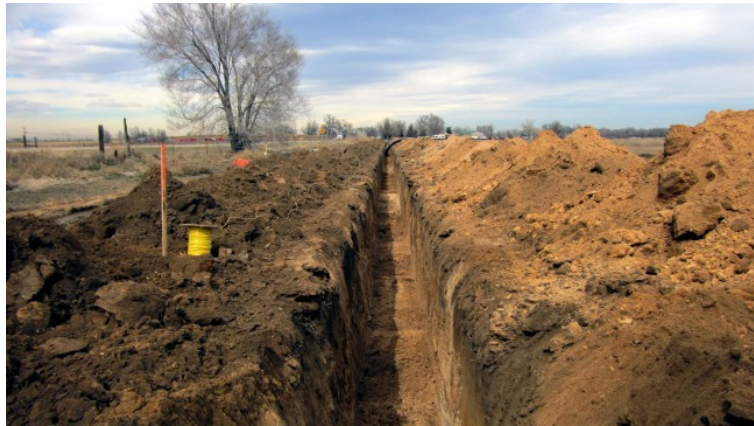
Trench for sub-surface produced water pipeline in Weld County Source: Colorado Public Radio, photo by Lesley McClurg, 2014
