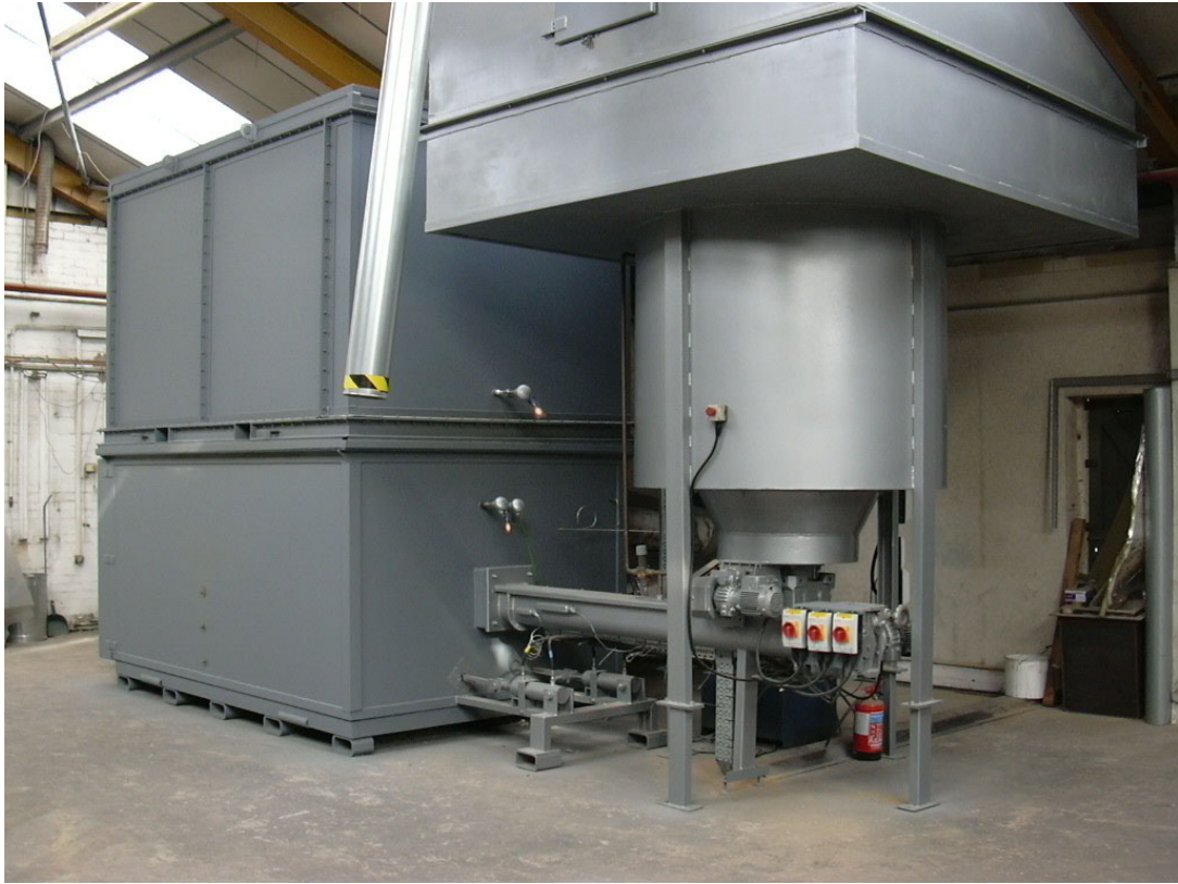
Fig 4.2 View of combustor from feed side
