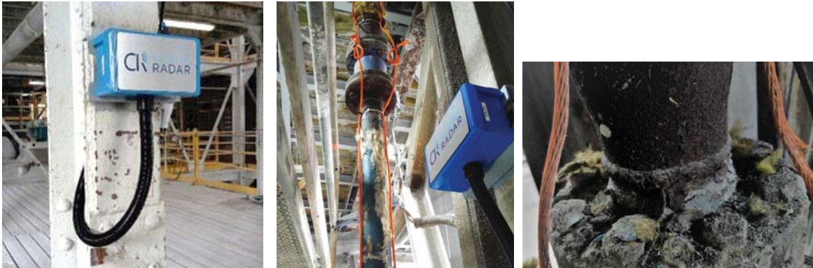
(Left) Field deployed unit, (Middle) Sensor on pipe surface, (Right) Corrosion located
