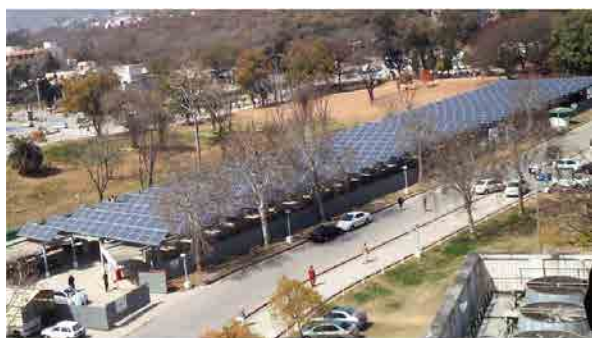
Solar System at PC
