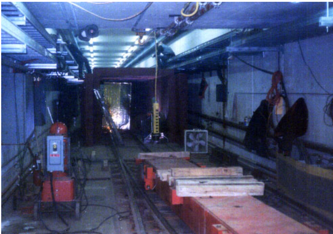
FIGURE 50. The NuTeV target “cave” under construction in 1995. The beam magnets were placed on carts which were rolled into place via the train tracks.
