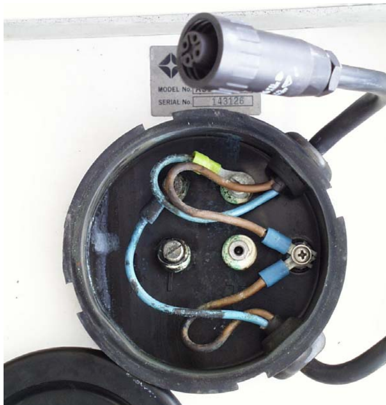
Figure 23: oxidation inside junction-box and detachment of one terminal.
