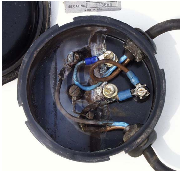
Figure 22: terminal oxidation (worst detected one).
