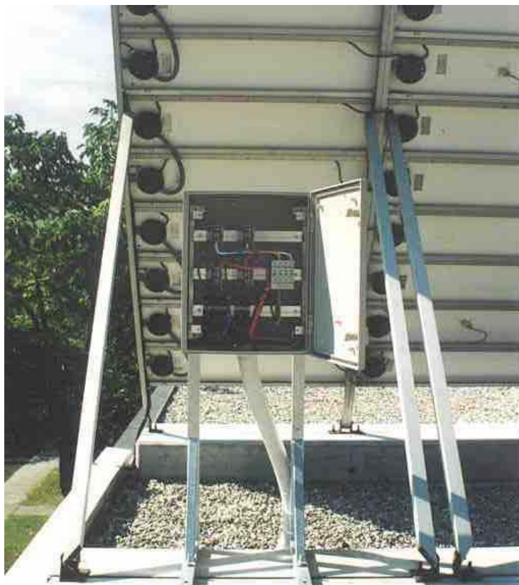
Figure 6: new field terminal box (1995).
