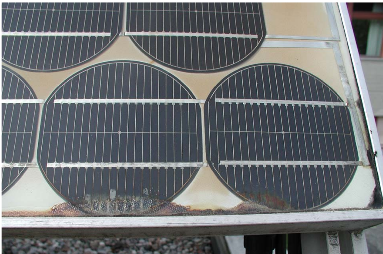
Figure 26: heavy delaminated module subjected to insulation test. No insulation failures detected.
