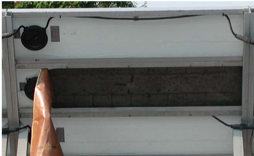
Figure 43: Tedlar detachment in modules subjected to 4000h DAH. After the test the module was installed in the plant, and complete detachment occurred after one year of further exposure.
