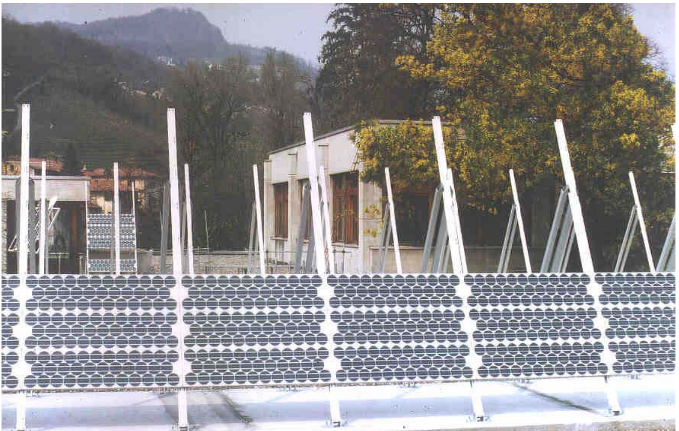
Figure 1: mounting structure of TISO 10 kW plant with some new ASI 16-2300 modules (1982).
